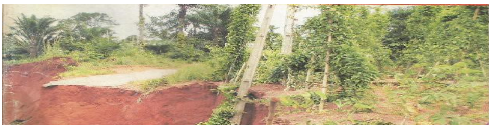
Plate 1c: Cutting of road by erosion Source: Field work, 2020
